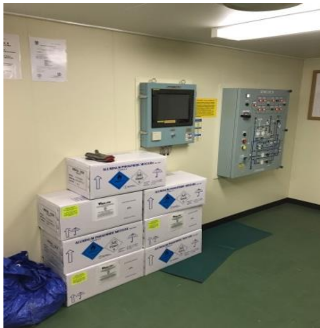
Improper placement and storage of the fumigant Weevil-Cide Pellets (PCP#: 30013)
